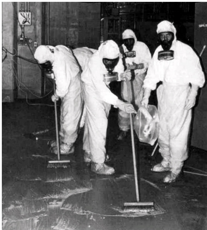
A clean-up crew works to remove radioactive contamination at Three Mile Island after the accident there in 1979.
