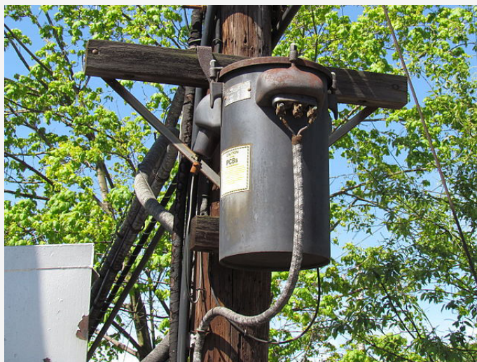
Old power transformers are a major source of PCBs.
