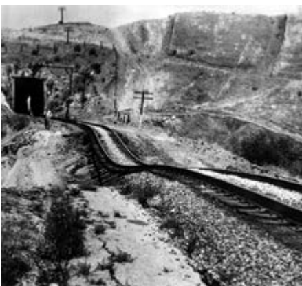
Damage caused by earthquakes
